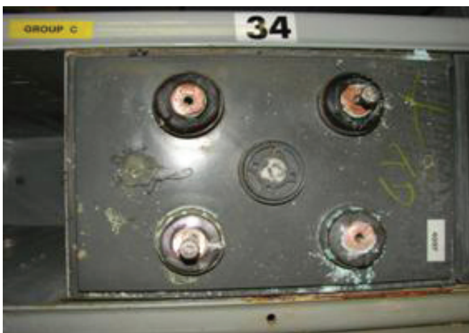
Figure 7. Terminal post corrosion was observed on several cells caused by electrolyte weeping through the cover bushing. The current carrying copper inserts remained undamaged.
